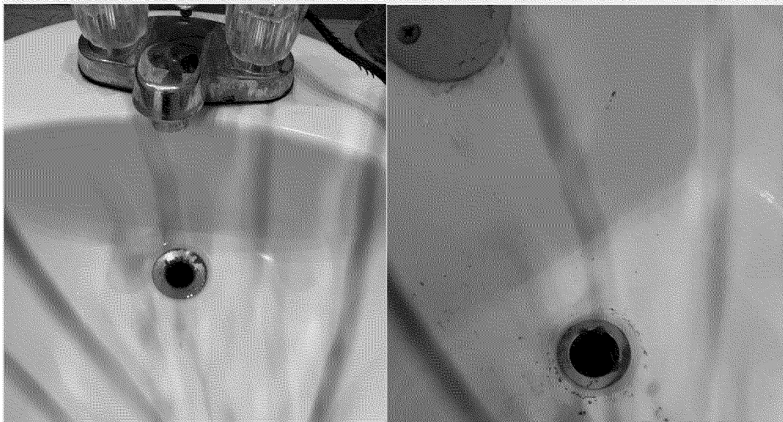
Picture 7. The broken sink and tub in the second-floor east bathroom.
