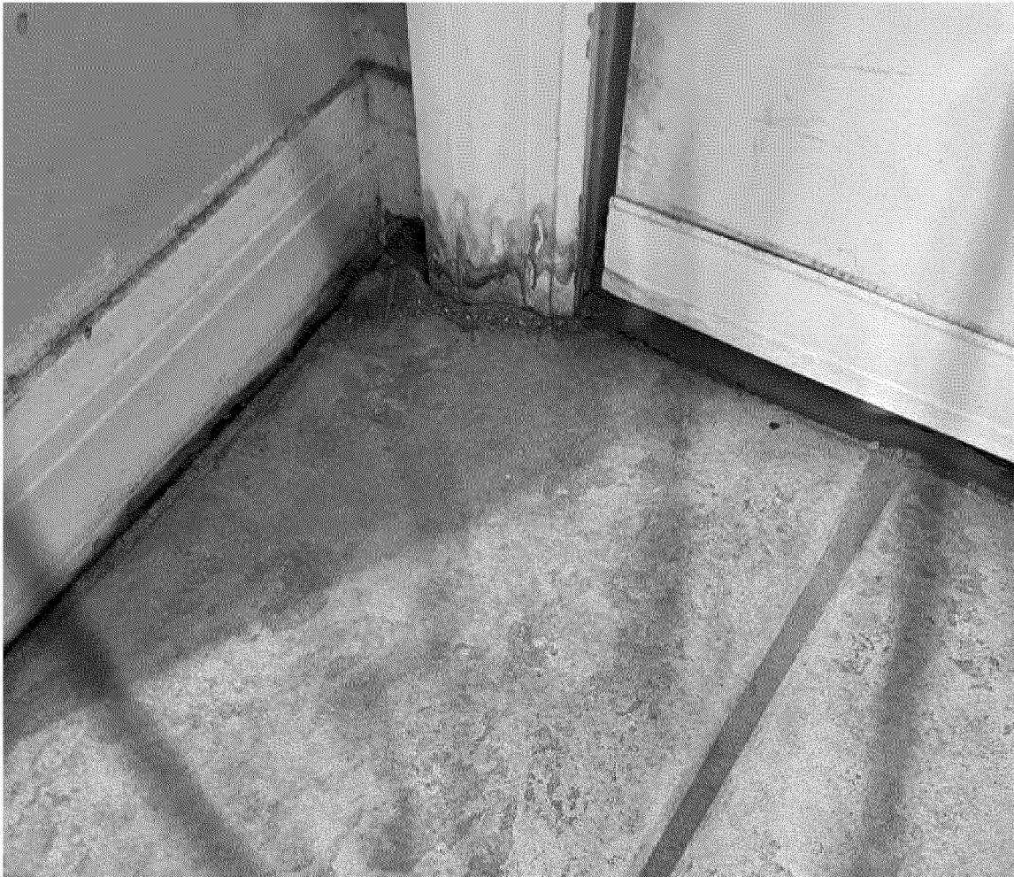
Picture 9. The rotten door frame with a hole.
