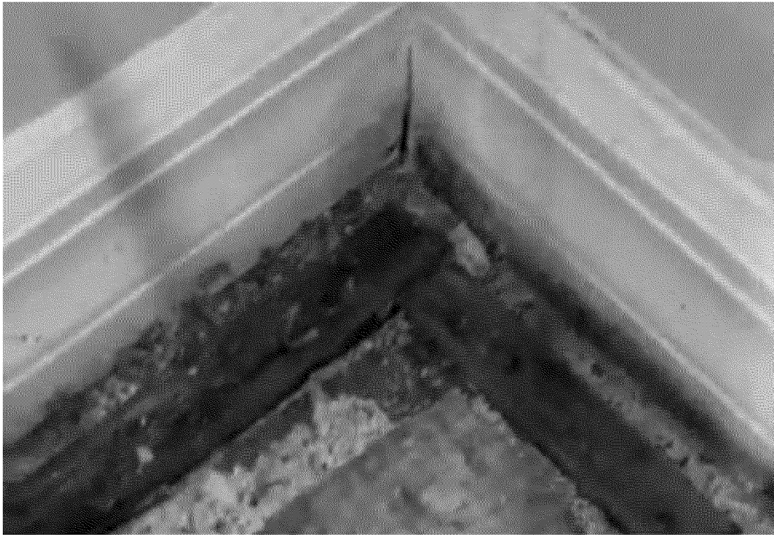
Picture 4. The decayed and blackened carpet tack strip and baseboard.
