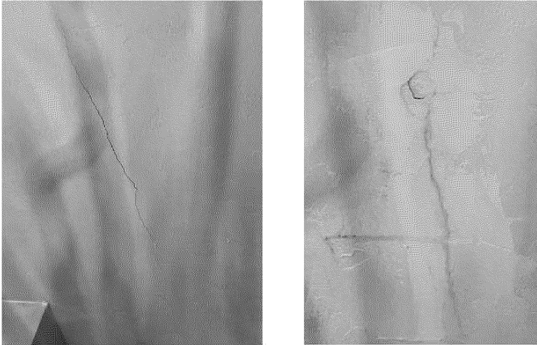
Picture 10. The original picture of the crack on the ceiling (left picture) and the fixed ceiling on August 24 (right picture). The replacement worker opted to address the issue by simply gluing the crack, a decision that was made with the landlord's approval. Unfortunately, this attempted fix proved ineffective, as the leak persisted.
