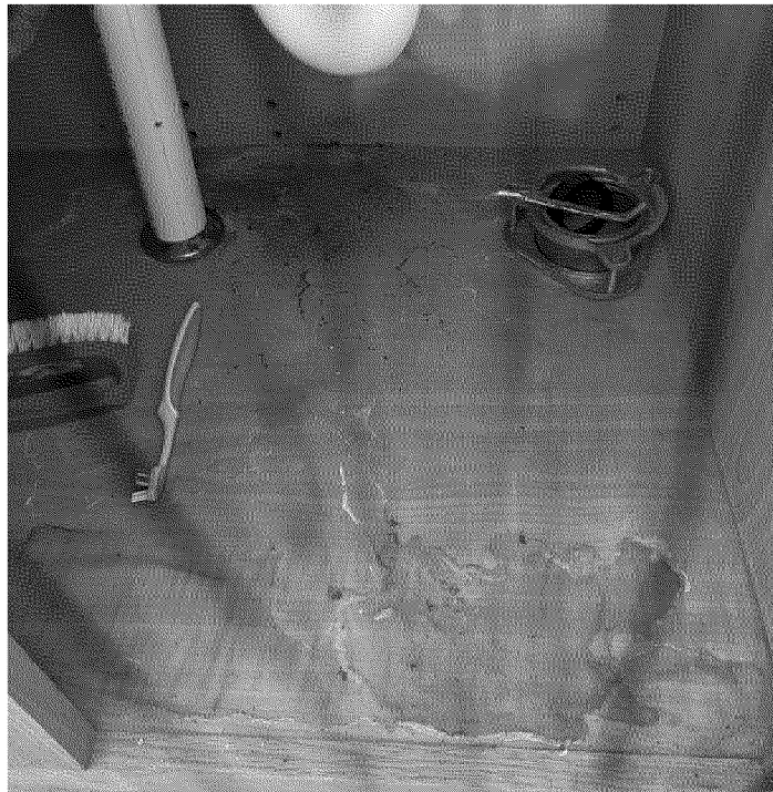
Picture 13. The leaking kitchen sinks.
